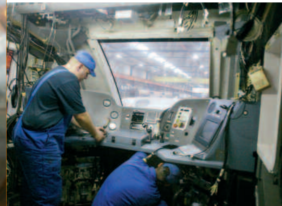
Right: Driver's desk being mounted in AGC set at the Crespin facility
